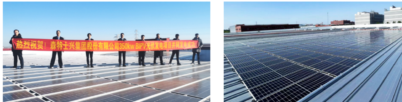
The photovoltaic power generation plant on the roof of the office building at Group headquarters and production base
